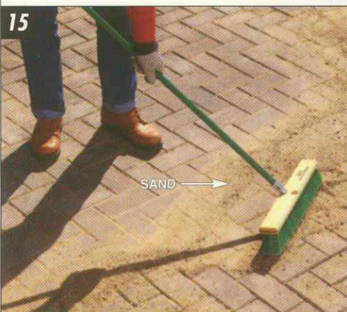
15 SWEEP COARSE, DRY SAND between cracks of pavers to lock them together and fill voids. Repeat with more dry sand in a few days.
