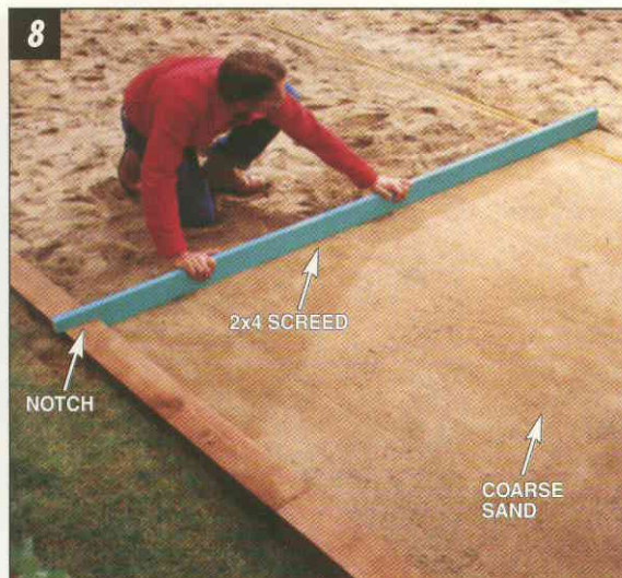
SPREAD AND LEVEL a 1-in. bed of sand over compacted subbase. Pipes provide a guide for dragging the 2x4 screed board across.
