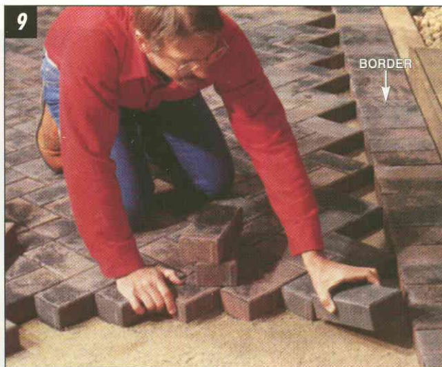
INSTALL THE PAVERS starting along the longest, straightest edge. Border pavers provide a crisp finished edge, especially along curved portions of patio.
