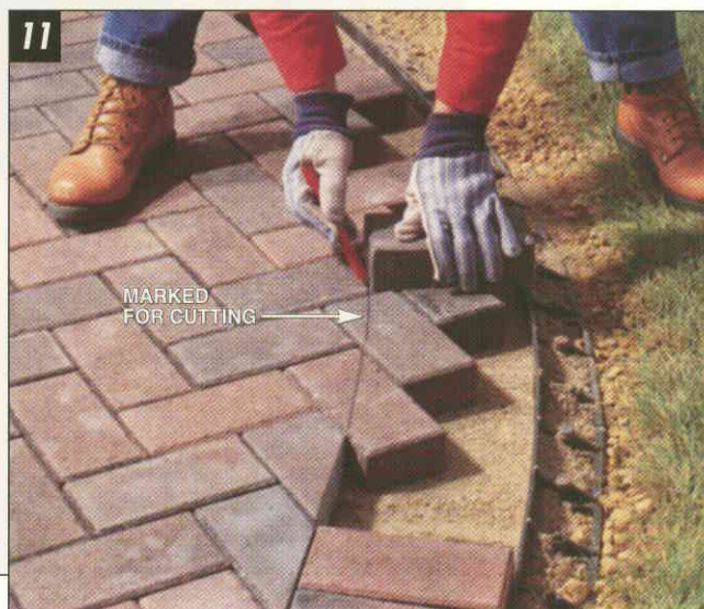
MARK PAVERS that run "wild" into the border area. Then remove the paver, cut to size and place back in position along with border paver.
