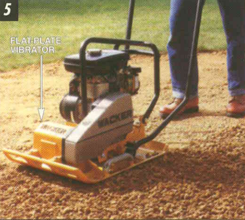
TAMP THE SUBBASE using a flat-plate vibrator (rented at $40 a day). Work in a circular motion and compact the area twice.
