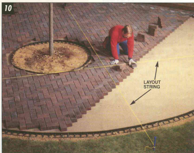
CONTINUE LAYING PAVERS using a layout string to keep them in line as you work. Put a gap between pavers or tap them tighter to stay in line.
