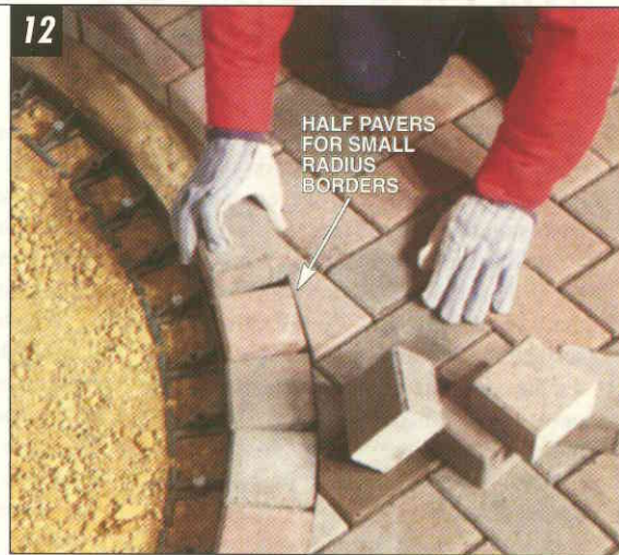
USE HALF PAVERS for bordering tight circles. Smaller pavers cut down on the size of the pie-shaped gaps between each piece.
